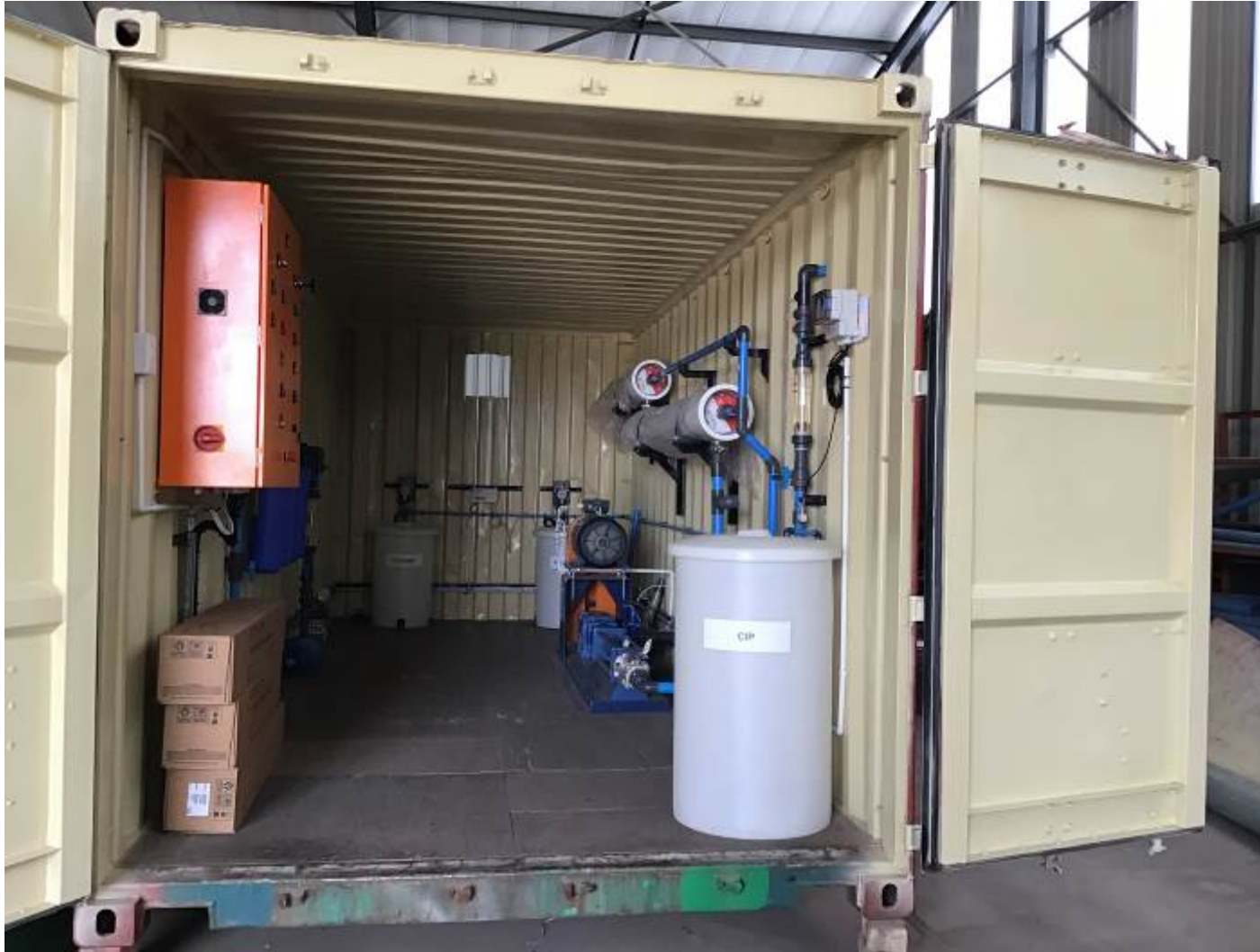
Picture 1: The desalination plant
